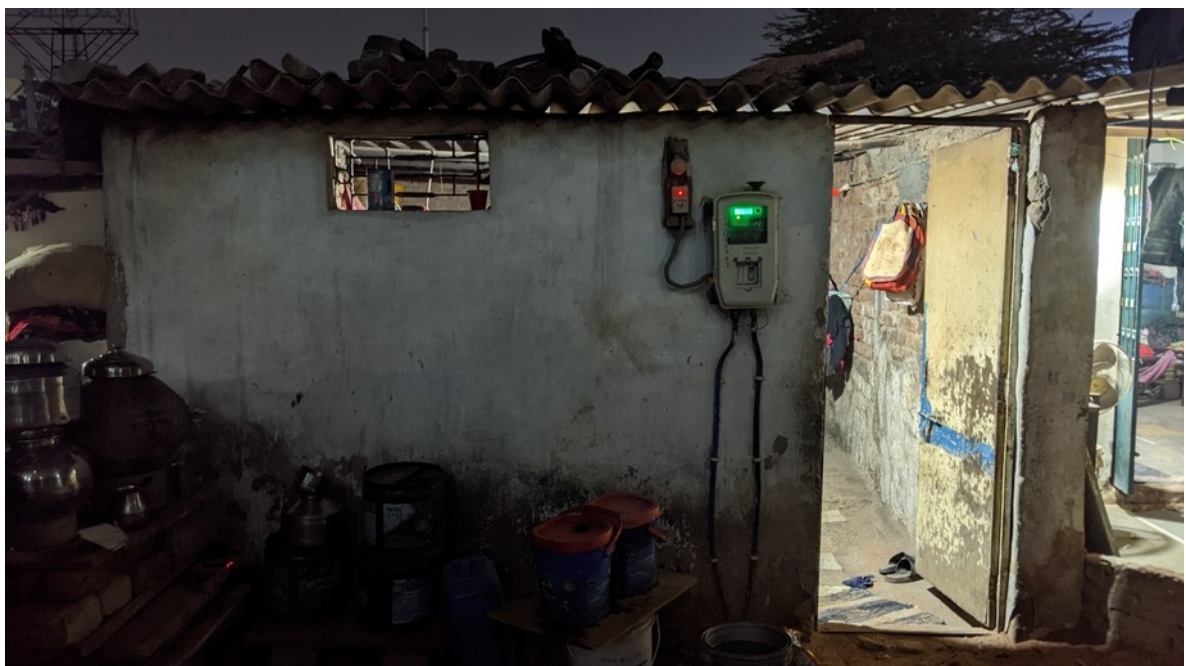
Figure 7: Electricity meter on a house in Sundervan basti; Source: Swastik Harish
